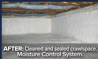
BEFORE: Damp, musty, moldy, hanging down and fallen insulation.
